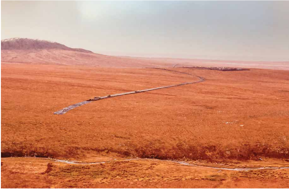
Building the 52-mile DeLong Mountain Transportation System (DMTS) haul road to the future Red Dog Mine in 1987.
