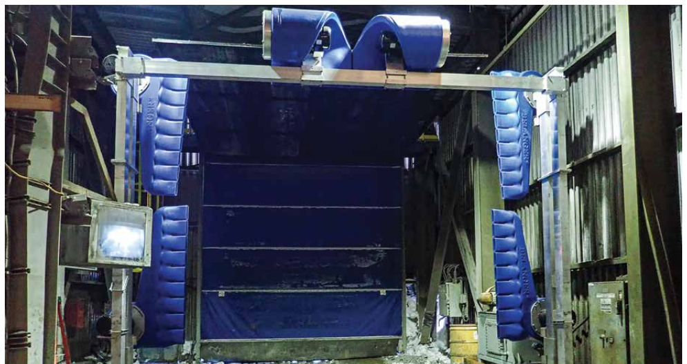
Red Dog is the first to install these unique air blades to remove any remaining dust from the haul truck as it leaves the offloading station. Instead of water, which can freeze up during the cold winter months, air is used at high pressure to blow the dust off the trucks before they exit the Truck Unloading Building (TUB). The dust is then collected by high-powered vacuums.
